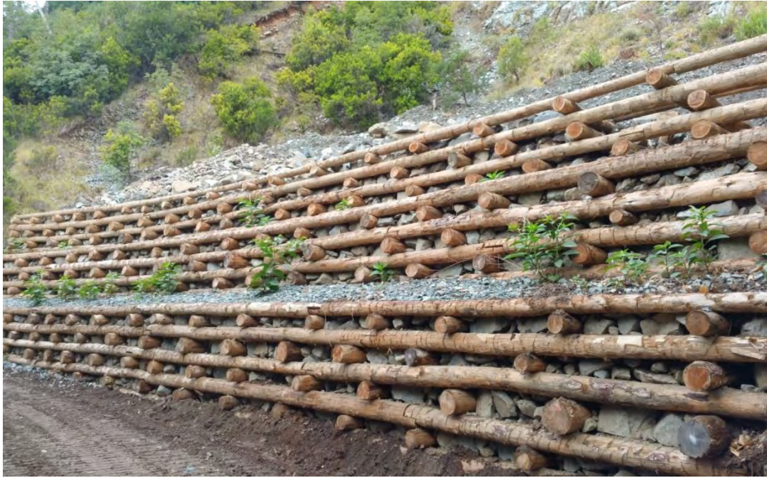
Figure 10.1: NBS solution applied for geological slope consolidation [Provided and owned by the Municipality of Genoa]
